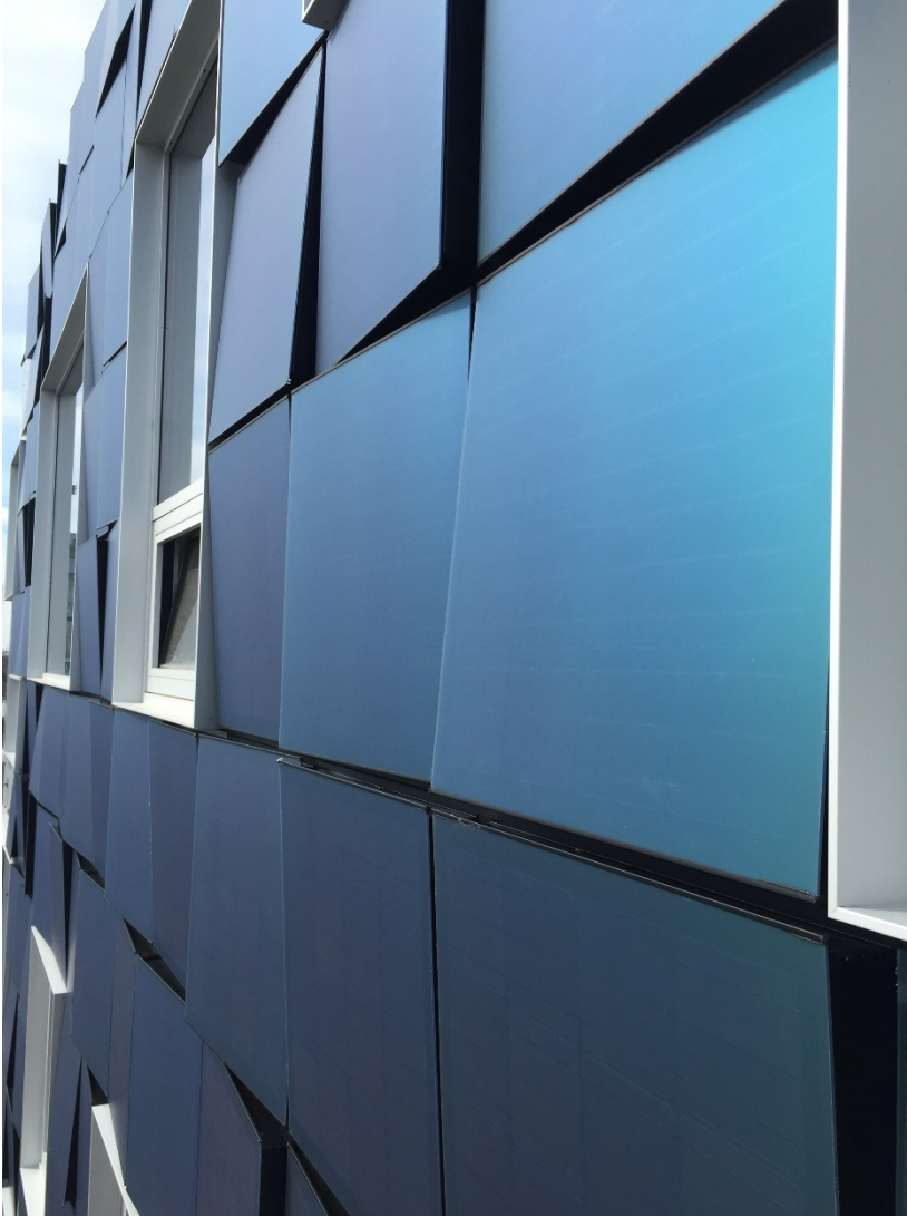
Figure 16: BIPV façade on Copenhagen International School (CIS) in Nordhavn, Copenhagen. Photo and installation provided by www.SolarLab.dk .
